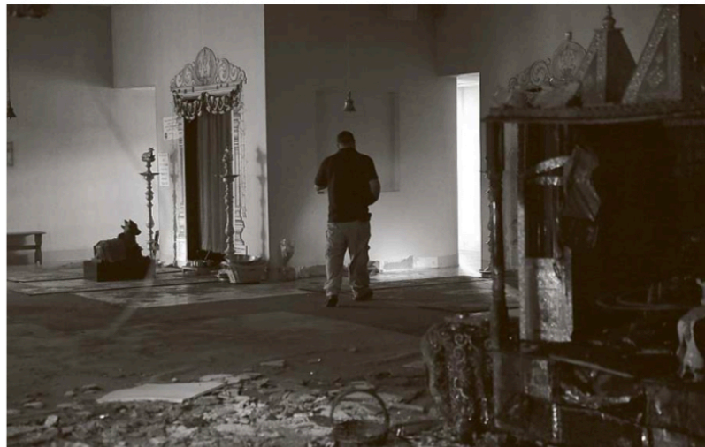
Geoff Mclear, a property manager for fire cleanup and restoration company Servpro, on Friday inspects the damage from a Thursday night fire at the Hindu Cultural Society of Western New York on North French Road in Amherst. Arson has been ruled out as a cause of the fire.
